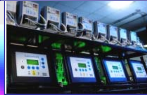
Regulators and I/O modules
